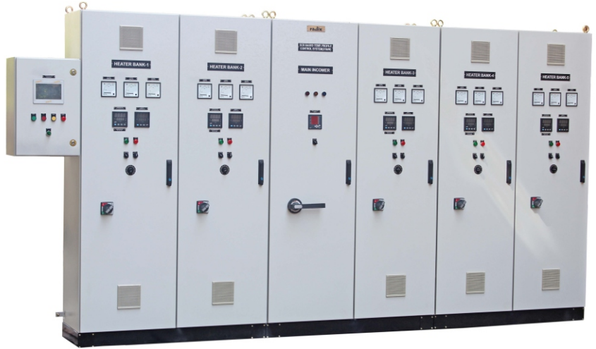
5-zone, 3-phase, SCR heating control panel Type of load : Resistive Capacity : 375kw Application : Multi zone - SS wire drawing annealing furnace
